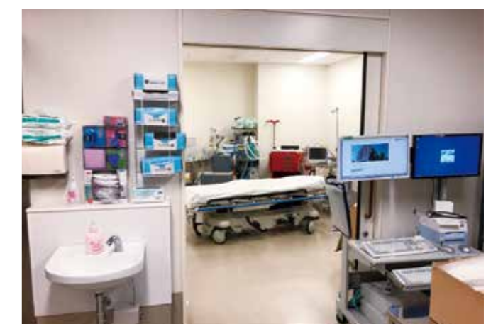
Photo 4 Negative pressure room. Patients suspected with COVID-19 have been basically treated in the negative pressure room installed in the ED. If the room is occupied, other two rooms are available for isolation purposes.
