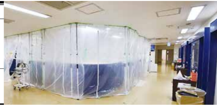
Installing positive pressure ventilation system in Nurses' station (Designation of Green Zone)
